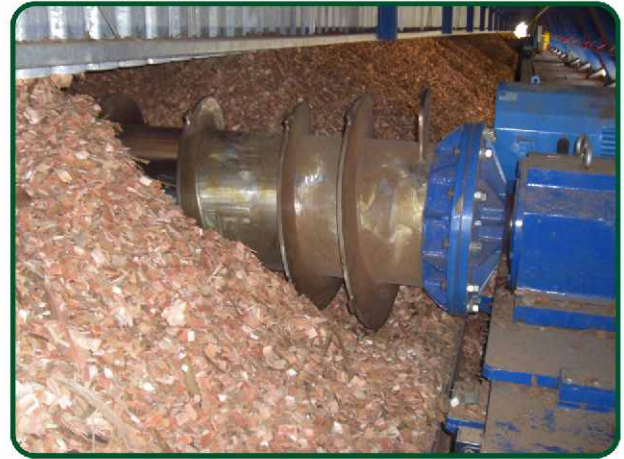
Biomass silo for 25.000m 3 loose storage capacity.
